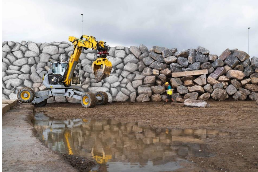
The Excavator picks and scans each boulder to be placed in the correct position. Circularity Park in Oberglatt, Eberhard AG. Credit: Marc Schneider, ETH Zurich
